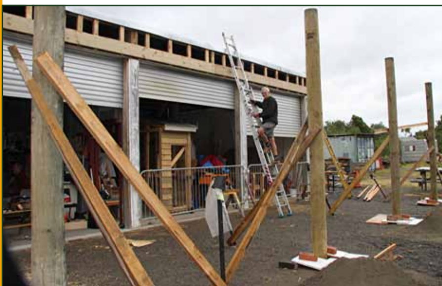
Peter Blackler working on the Kapiti MenzShed expansion, building a verandah to enable more work to be undertaken wet or fine.
