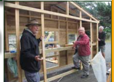
Kapiti MenzShed members are building a 'house' for the local Montessori group.
